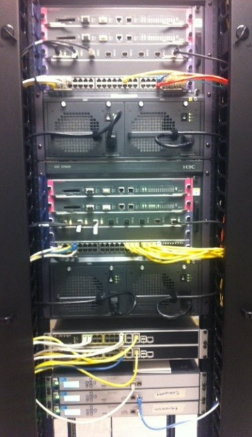
New Core Switches building
